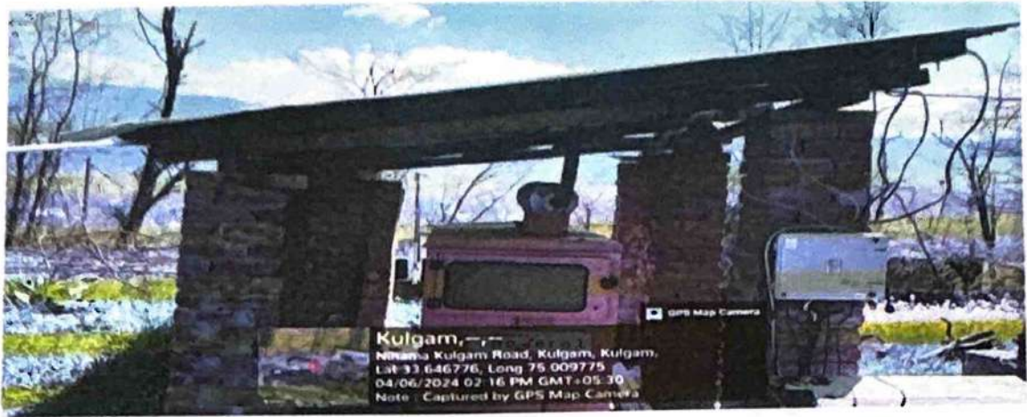
Fig.3: Genset facility of the college
