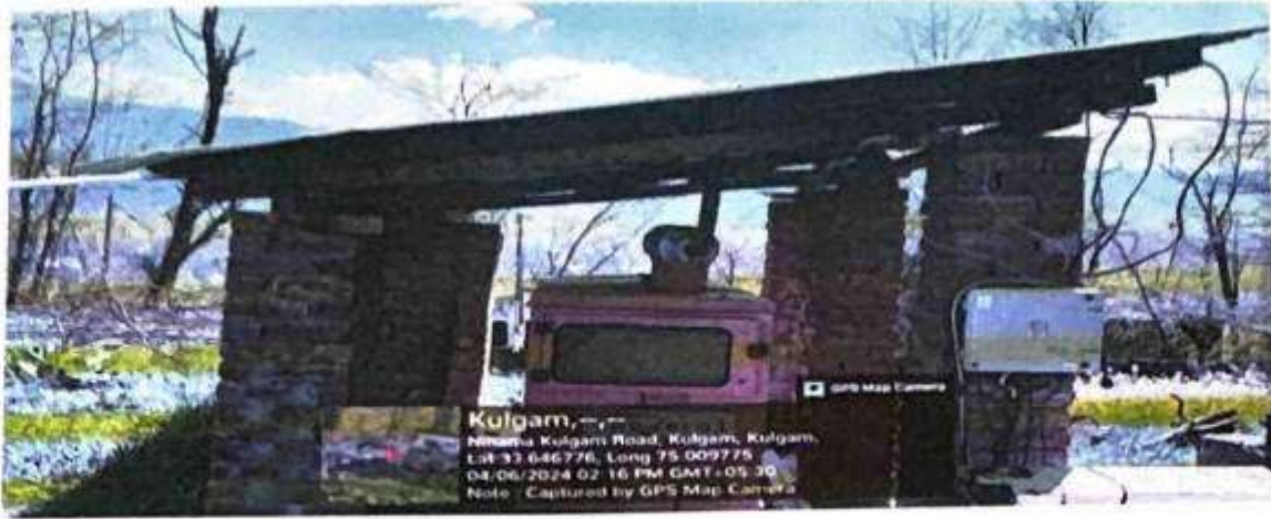
Fig.3: Genset facility of the college
